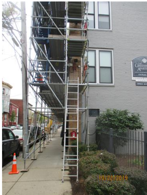
Access Ladder violations (2)
