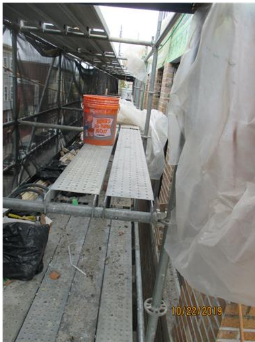
unplanked platform/debris area
